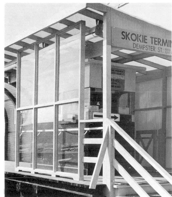
Transparent plexiglass windscreen installed to protect the fare collection area at Dempster terminal. Between 2,000-2,800 persons pass this booth each weekday morning between 6:00-9:30 a.m.
