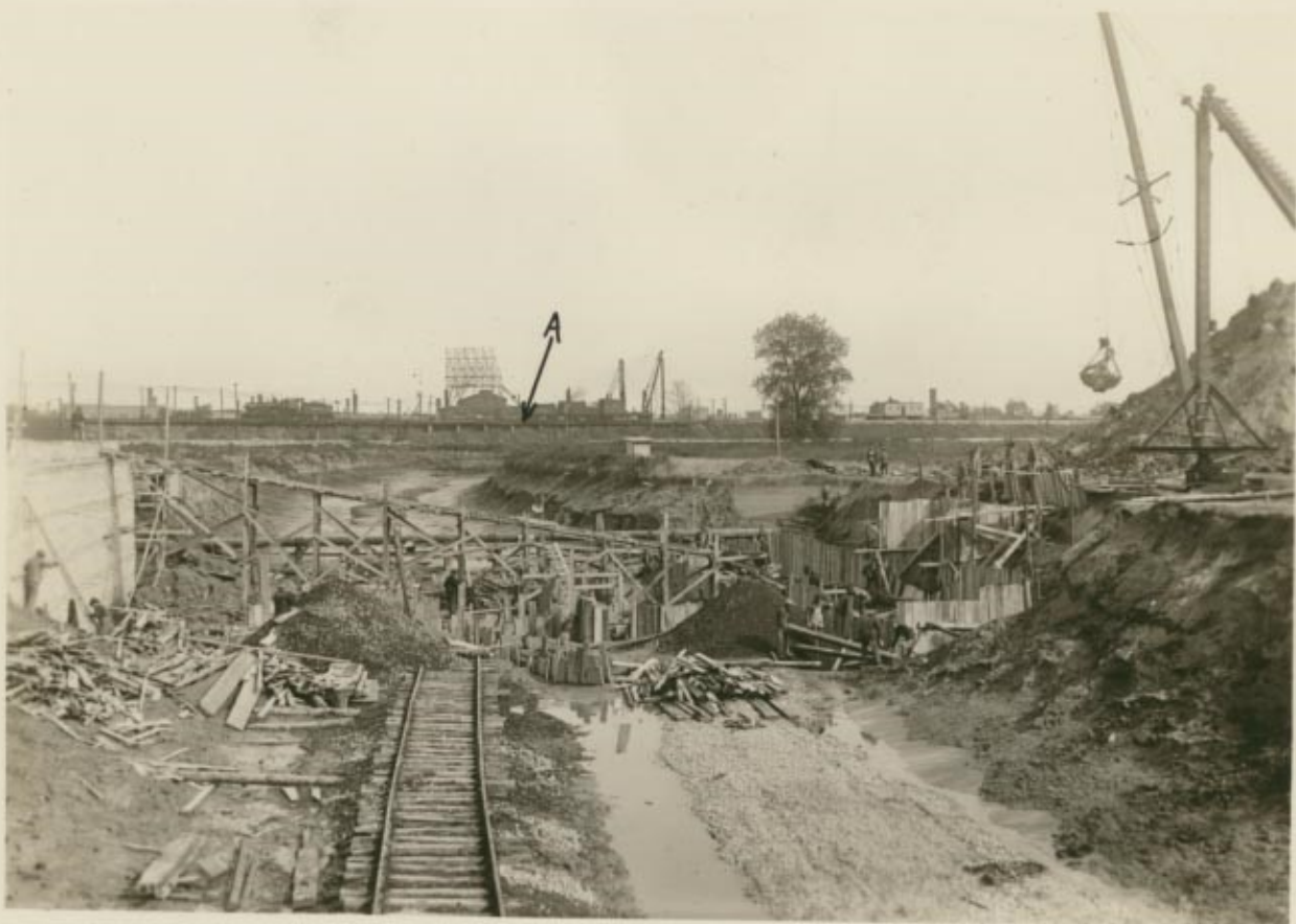
Looking east September 30, 1924 from the future Custer Street bridge, on the Skokie Valley Line, and showing a section of the roadbed, which at this place averages about 12 feet in depth. At the point marked "A" the new line will pass between the main line of the Milwaukee division of the Chicago and Northwestern railway, and a crew may be seen driving piles preparatory to beginning construction of the subway. In the foreground are construction facilities for the Custer Street bridge over the new line.
