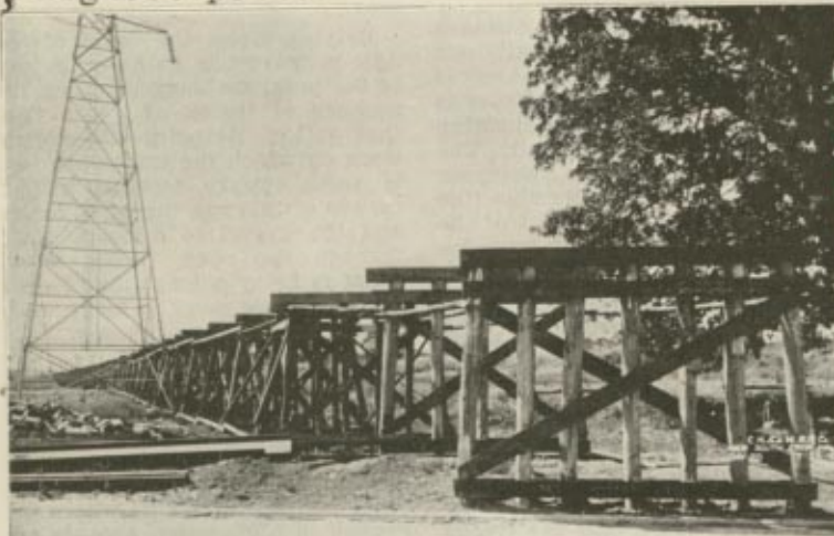
Trestle work at low spot on Skokie Valley Division, North Shore Line
