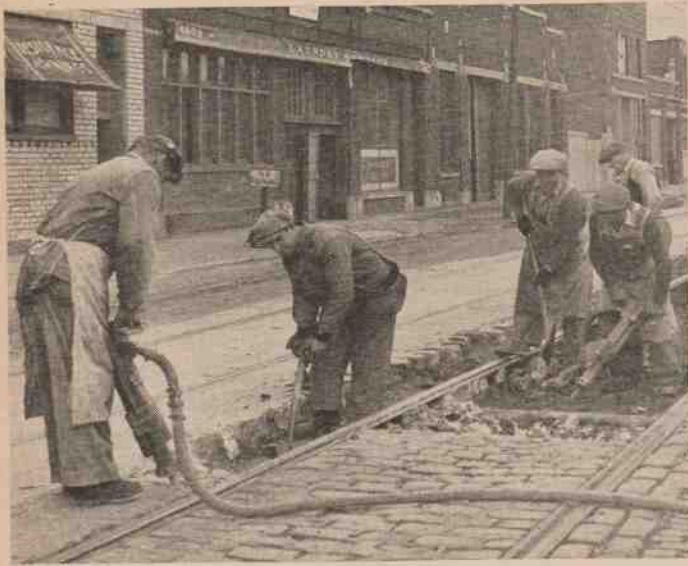
THE BREAKAWAY: Pneumatic paving breakers are used to dig out paving blocks and break up the concrete paving foundation, thus exposing the rail, fastenings and ties. After base of the rail has been exposed, the ties are tested (and replaced if necessary), rails renewed, surfaced and aligned, and new fastenings installed. The concrete paving foundation is then replaced and the track is ready for paving.
