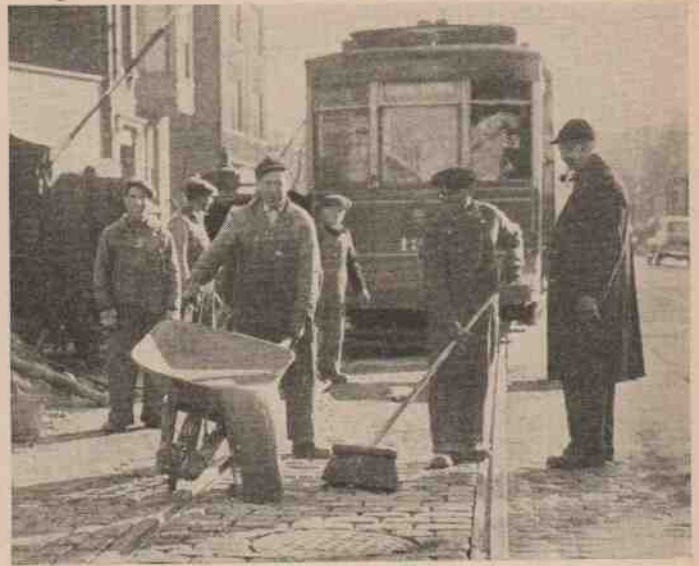
THE SMOOTHING: In paving the track, a bed is laid consisting of a layer of torpedo sand about 1 1/2" deep, and the paving blocks are then laid on this bed. Paving block is then covered with a thick grout (mixture of cement and sand) which is thoroughly broomed into the openings between the blocks and into the space under the head of the rail, and allowed to set.
