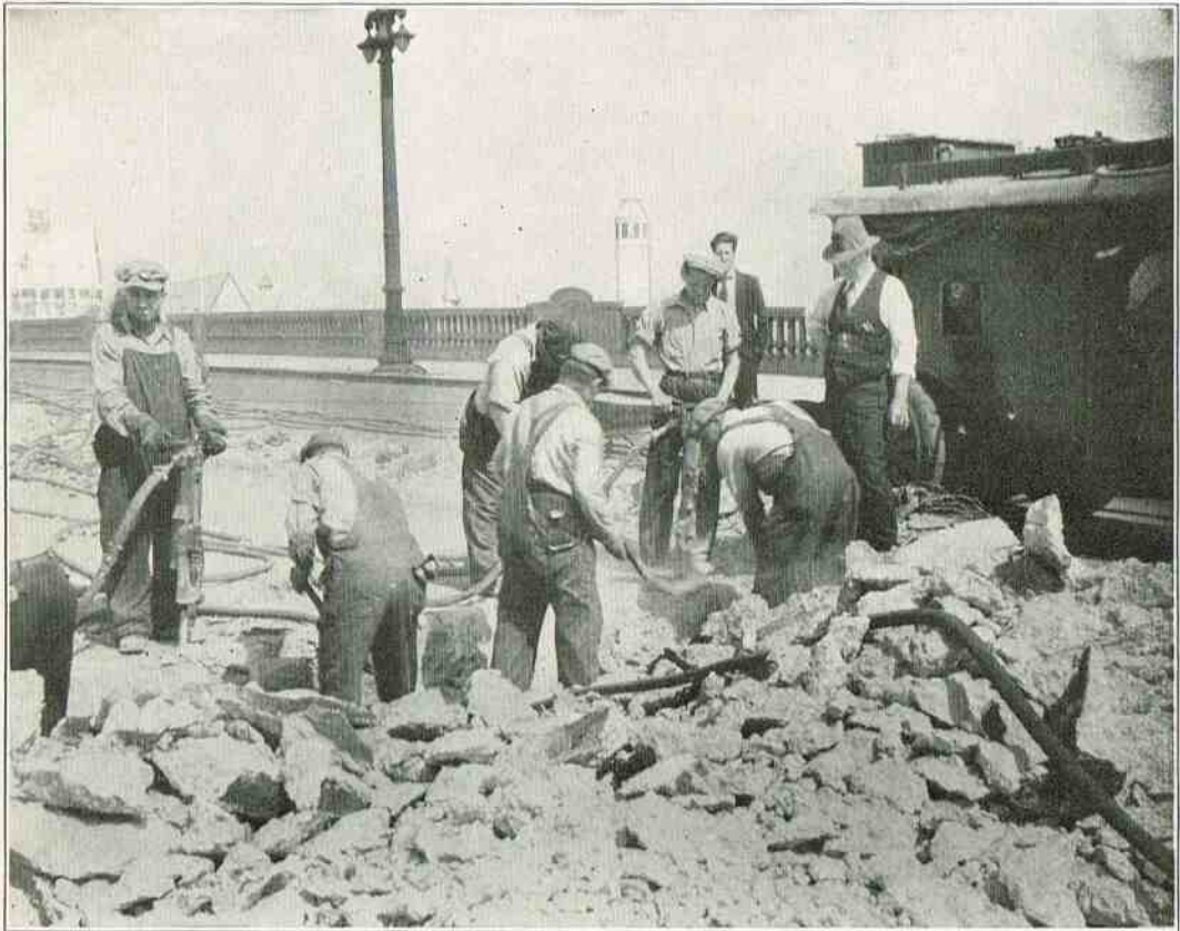
Knee Deep in Concrete at the West End of 23rd Street Viaduct
